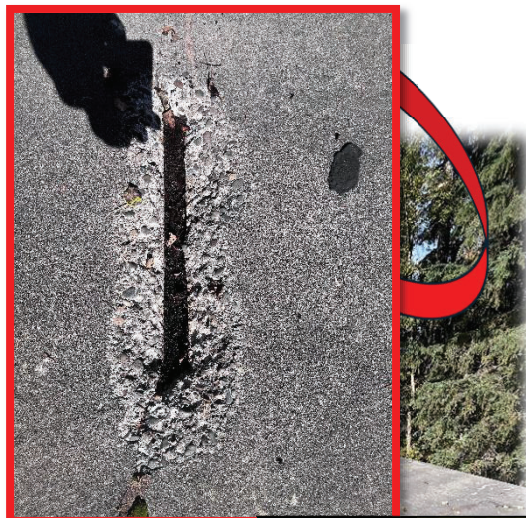
Benjamin Reservoir lid concrete spalling (repaired in 2025)
