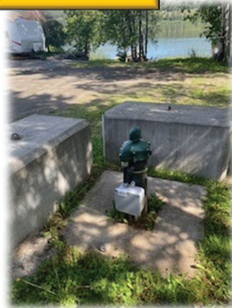
Horse Lake Wellhead
